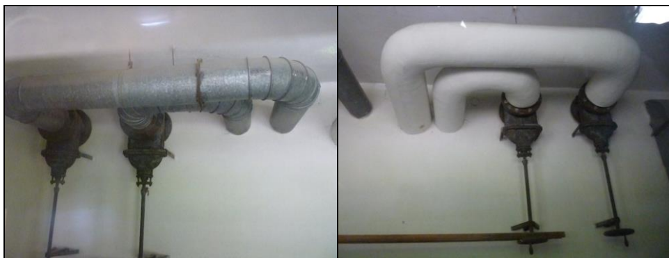
III. 24: Thick pipes in the room behind and in the area above the Dachau “gas chamber.”
