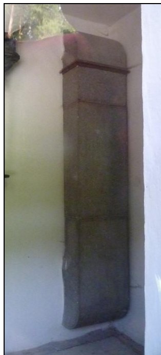
III. 26: Warm-air-supply shaft behind the Dachau gas chamber.
