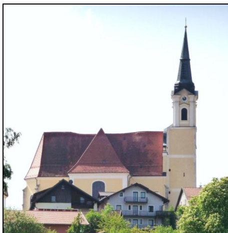
III. 84: In 1972, the Catholic church in Untergriesbach, Bavaria, was fumigated with Zyklon B. Subsequently the entire plaster turned patchy blue (Konrad Lackerbeck; Wikipedia commons).
