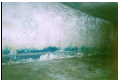
III. 89: Zyklon-B delousing installation, Chamber III (east wall), of building 41 in Majdanek. (© C. Mattogno)
