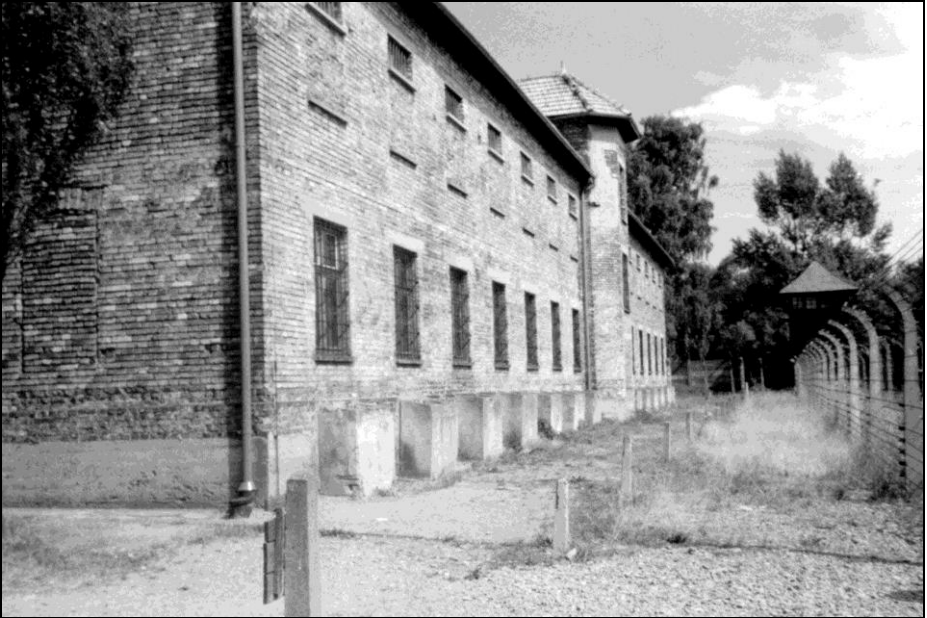
Photo 26: Block 11, outside, wall facing SSW, concrete screens around the window wells of the bunker cells.
