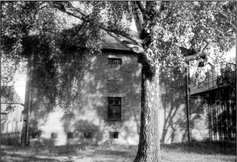
Photo 29: Block 11, outside, wall facing SE, sheet-metal boxes covering the air-supply holes of the 4 stand-up cells (Stehzellen) of the bunker. In the center underneath the large window: window of cell no. 21 (see Photo 17).
