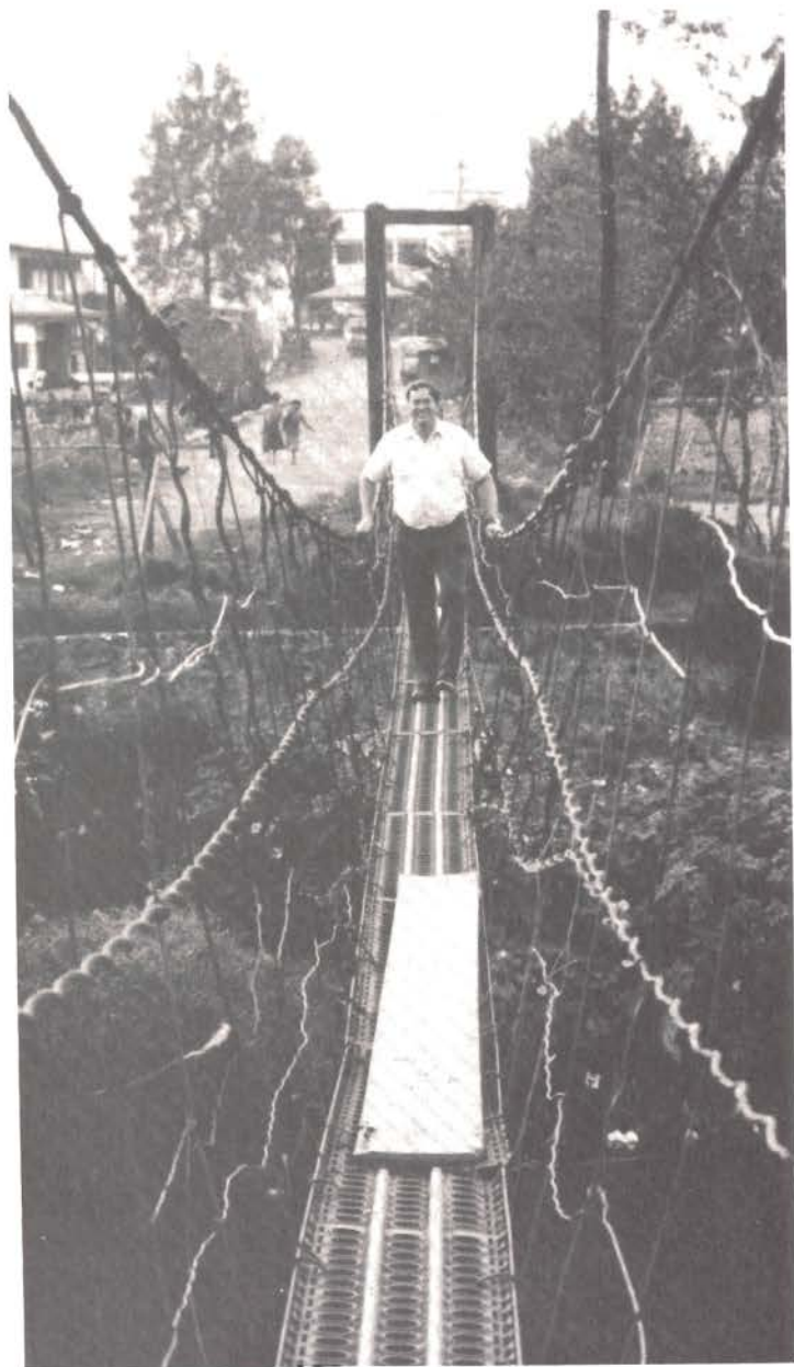
In countries which have a lot of creeks and small streams, a suspension bridge like this one can easily be sabotaged.
