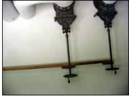
III. 10: Heavy insulated hot water (or steam?) pipes in the room behind the alleged gas chamber of Dachau leading into the space above the current room. 35
